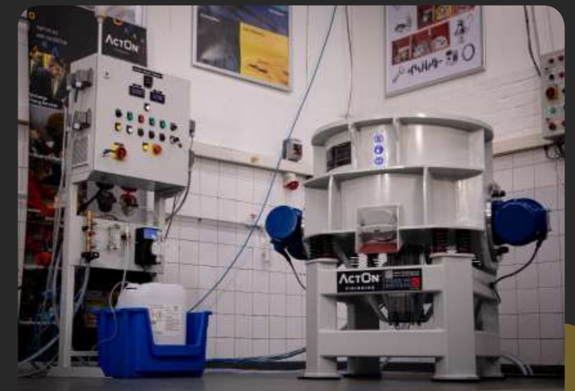
AWP188P system with control panel and dosing unit
